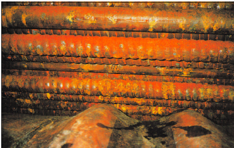
Photo 2.4 Corrosion of a fire and flue-tube boiler by dissolved oxygen
